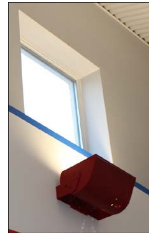
Figure 10. Main Corridor Fixture
